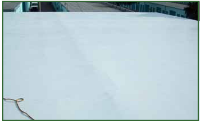
The finished roof is a durable, white, heat reflective, energy-star rated system with CIRSCO's 2-year warranty.
