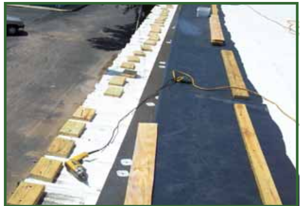
New treated wood nailers are installed around the complete perimeter of each roof area.
