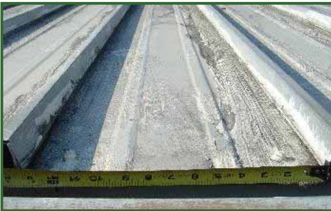
All fastener issues and rust must be treated
