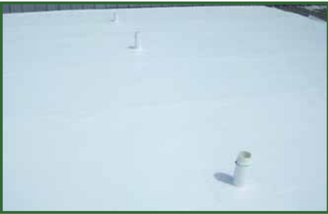
All roof penetrations are “flushed” with the same material heat-welded to the membrane.
