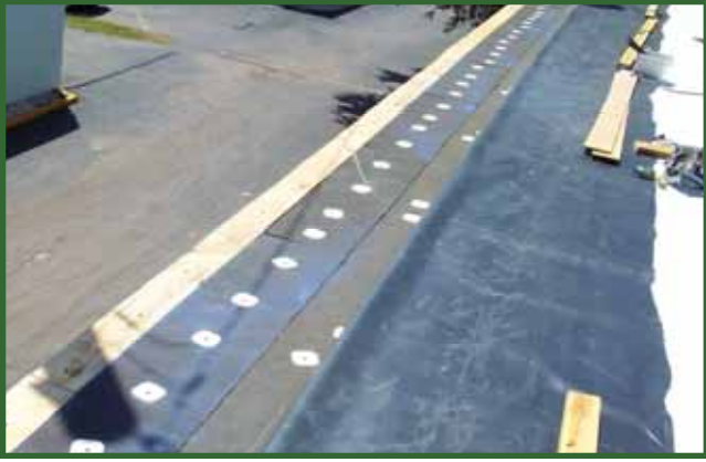
The treated wood is attached to the structural components to serve as anchors for the finished metal.
