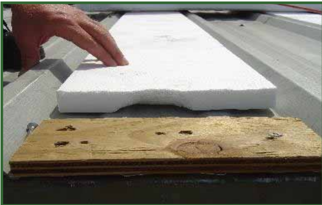
"Flute-filler" insulation is installed between the rib sections of the metal panels
